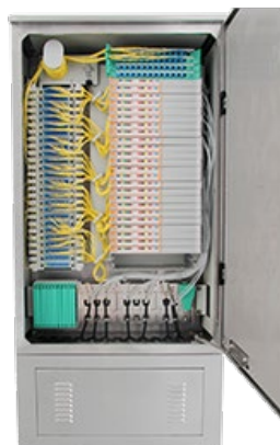
Figure 5. Optical Distribution Cabinet (ODC)
